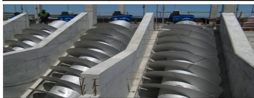
Archimedes-type screw water pump of some 3 m diameter - the UTCLT project would need bigger diameter.
