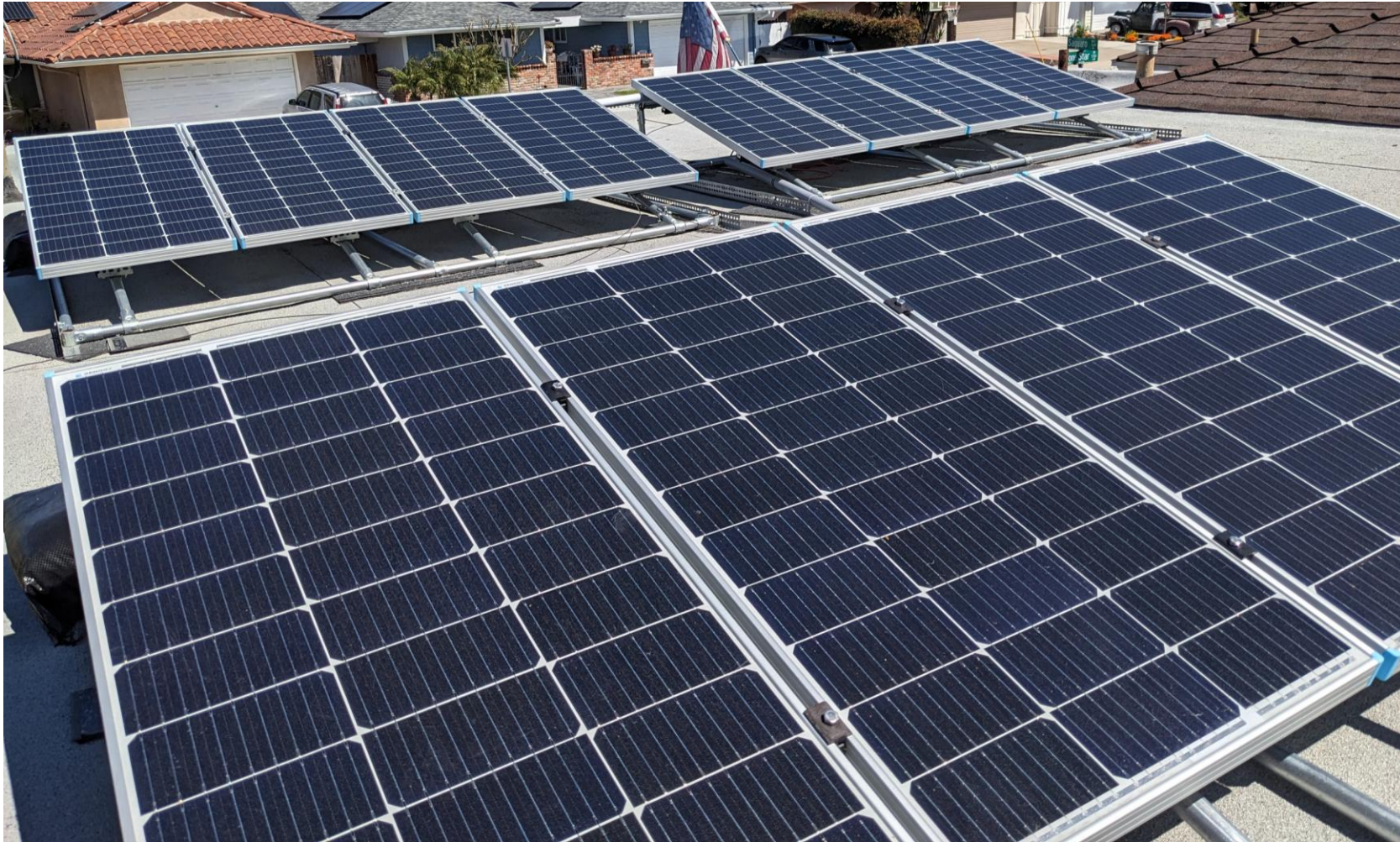
Completed 1200 Watt relocatable solar panel array
