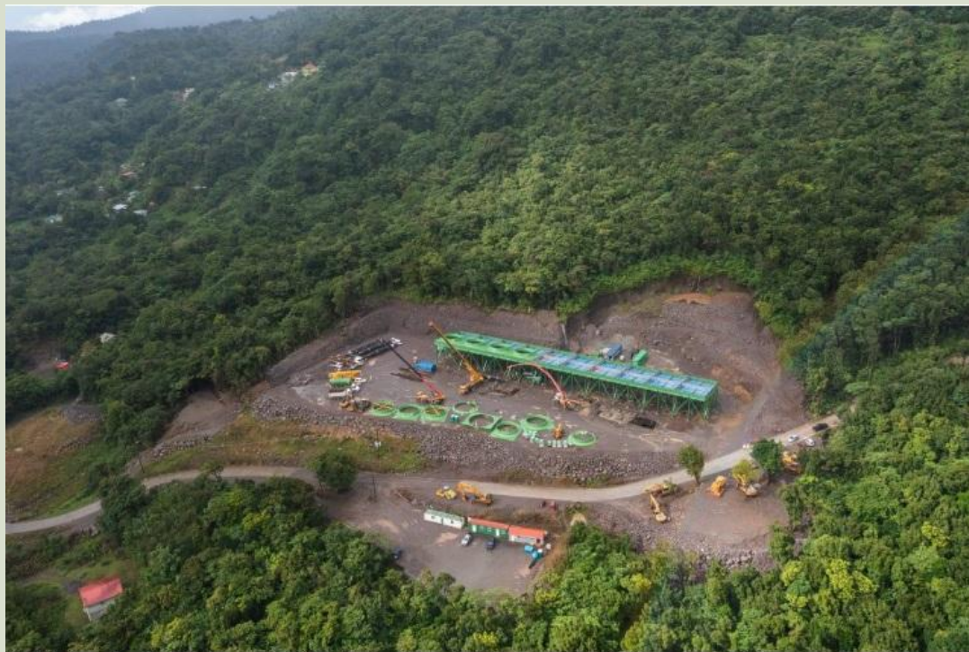
Aerial view of construction work at the Dominica geothermal power project (source: PM Roosevelt Skerrit)
