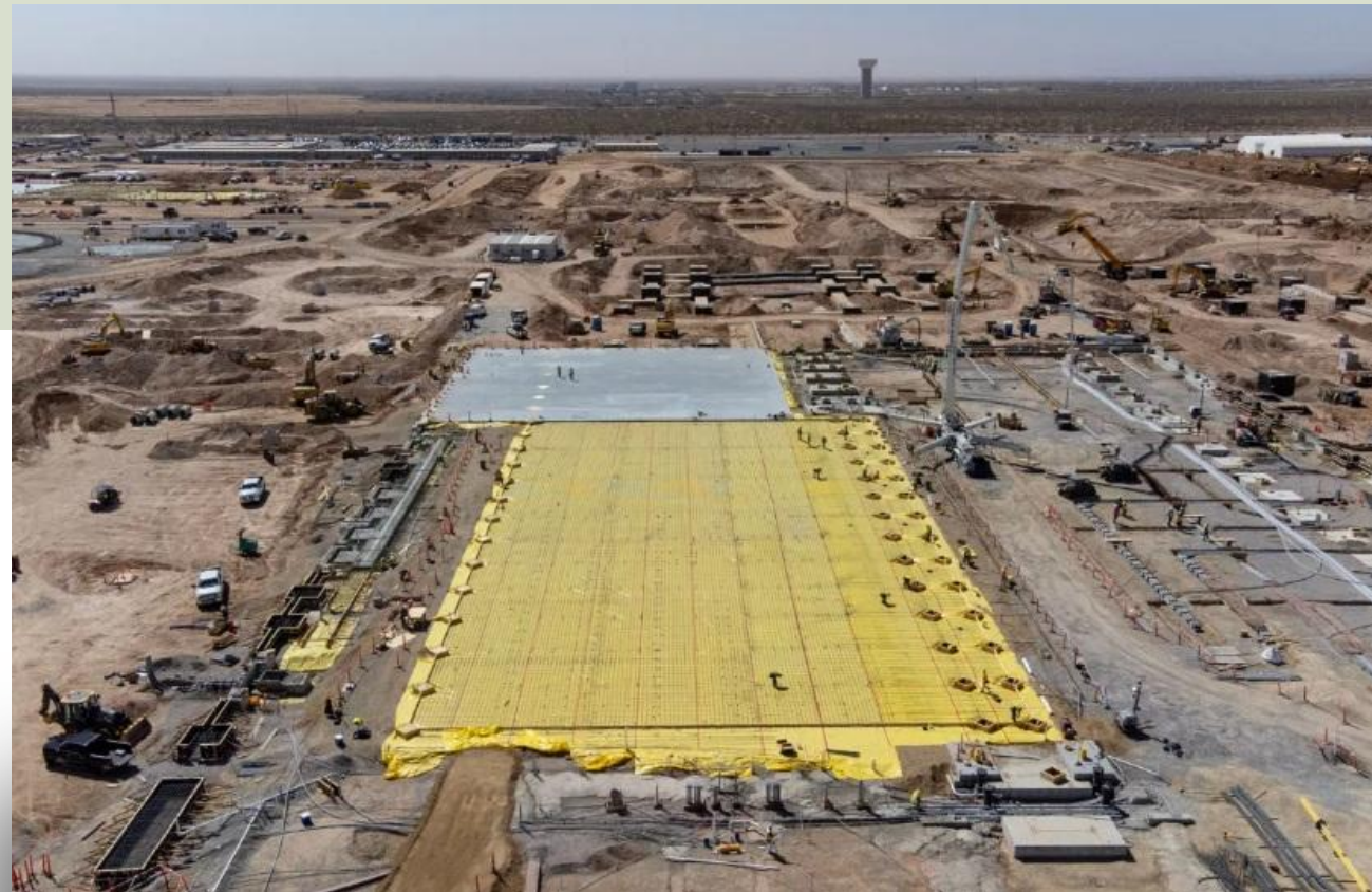
Meta Platforms data center complex on a 1,000-acre site in far Northeast El Paso. Omar Ornelas/El Paso Times/USA TODAY Network via REUTERS
