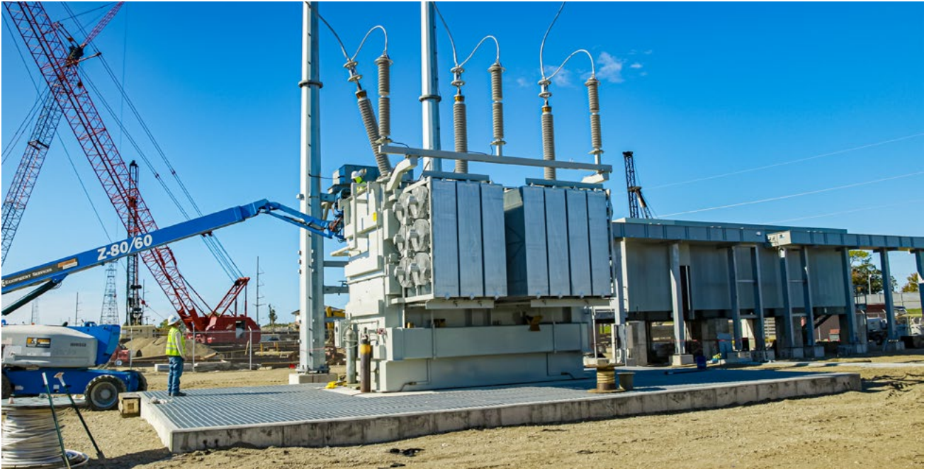
The team moved quickly to purchase the 230/24 kV 67MVA transformers in 2022; they were delivered a year after purchasing. The transformers feed the 24kV enclosed bus duct connecting to the 24kV Switchgear on raised foundations for flood mitigation. Transformer lead times are now significantly longer than what was seen in this project.
