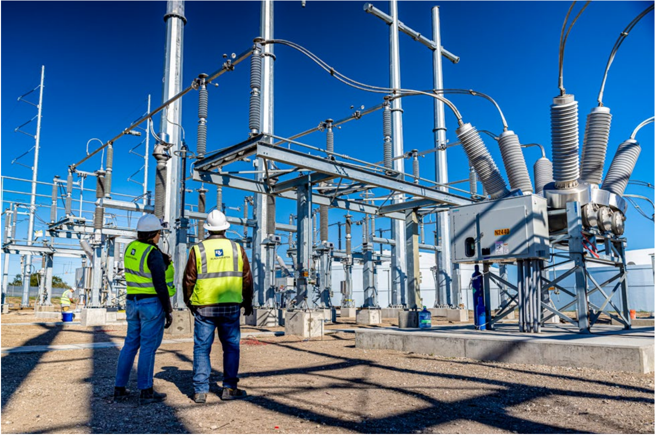
On the right of picture, 230kV HV breakers, which required collaborating with the client to allocate breakers for other projects to ensure were delivered on time. The equipment took a year to deliver after purchasing - now lead times over 2 years.
