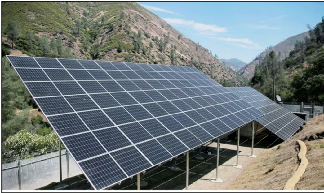
A solar array built by BoxPower 2 is charging batteries and keeping five PG&E customers supplied with electricity at a remote grid project in Briceburg, California. (BoxPower)
